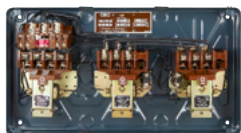
Interior View of MK2 SASD
