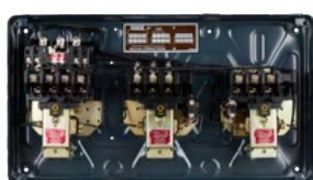
Interior View of MK1 SASD
